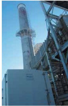
Continuous emissions monitoring systems.
